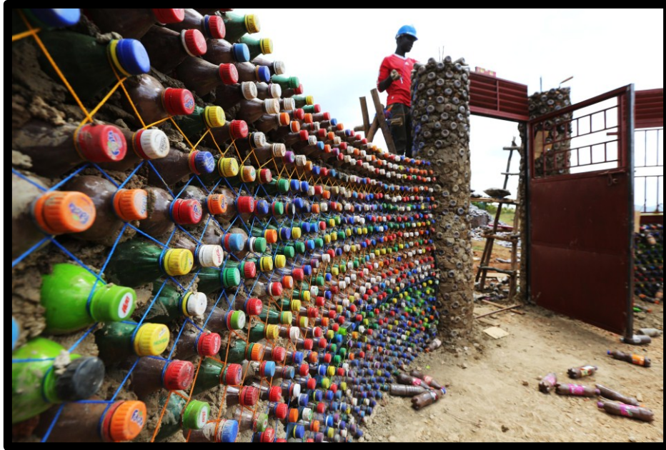
Figure 3: Plastic bottle upcycling construction of the first learning hut at SINA (image taken by the author)
